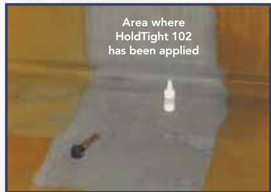
Above: View inside a tank where HoldTight 102 was applied to a panel. Note the flash rust that has appeared on the untreated area. The treated HoldTight 102 area will remain rust free for up to 48 hours or longer after application.
