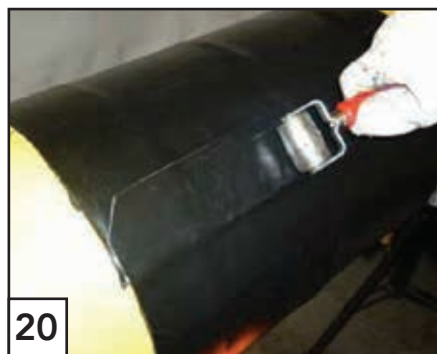
20 Roller the closure patch in the overlapping area. Let the installed closure patch cool down before continuing with application.
