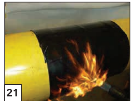
21 Beginning below, heat the middle of the sleeve, moving the torch in a circumferential direction with blue-yellow flame. Use the same motion to shrink one side, then the other side. Ensure even shrinkage.
